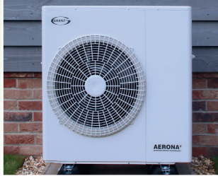
Air Source Heat Pumps / Electric Storage Heaters
